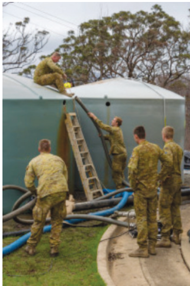
Australian Army soldiers connect hoses to a Bega Valley Shire Council water tank while installing an Army water purification and desalination system to supplement Bega Valley's drinking water supplies during Operation Bushfire Assist 2019-2020. [Photo: Sergeant Andrew Eddie, Department of Defence]
